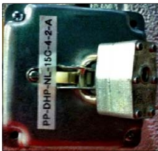
SAMPLE OF DISCONNECT SWITCH
